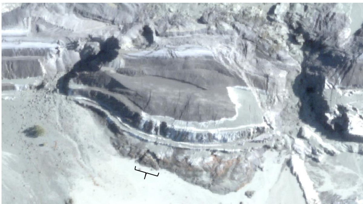
FIGURE 43 EVIDENCE OF SLIDING ON THE BASE SUGGESTED BY BLOCK SEPARATING FROM EMBANKMENT TOE (CURLY BRACKET).
