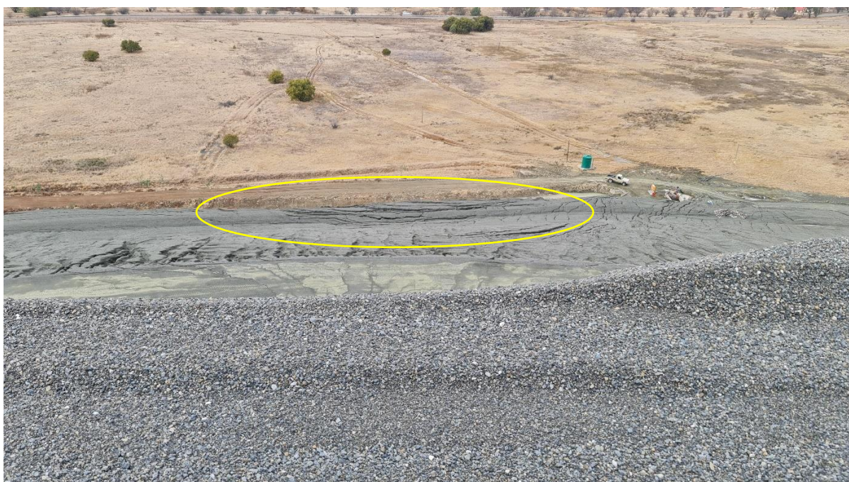
FIGURE 7 CIRCLED AREA HIGHLIGHTING TRANSVERSE CRACKS ON THE SOUTH-EASTERN WALL WHICH MAY BE INDICATIVE OF SUBSIDENCE TOWARDS THE DOWNSTREAM TOE OF THE DAM WALL. THE CIRCLED AREA COINCIDES WITH FAILURE SCAR 3. COMPARE TO SATELLITE IMAGE B23. (DATED 27 JULY 2022.)
