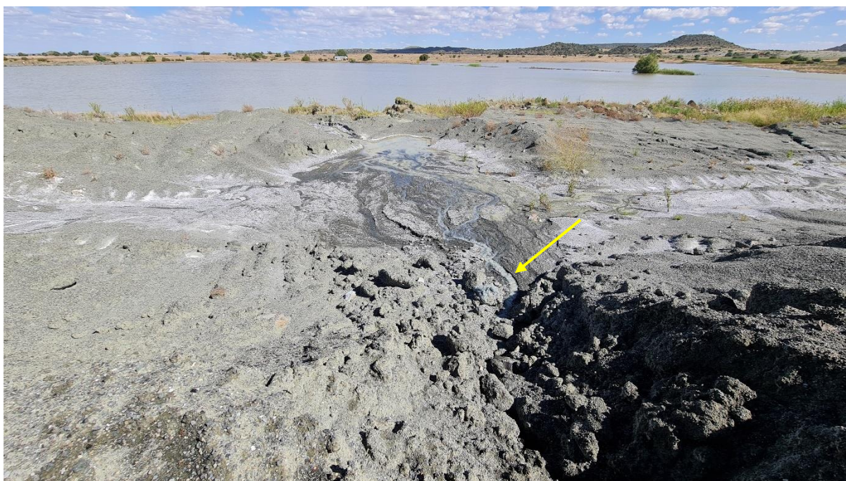
FIGURE 6 TURBID SEEPAGE WATER EMERGING FROM THE TOE OF THE TAILINGS DAM OPPOSITE DAM 10. (DATED 28 MARCH 2022.)
