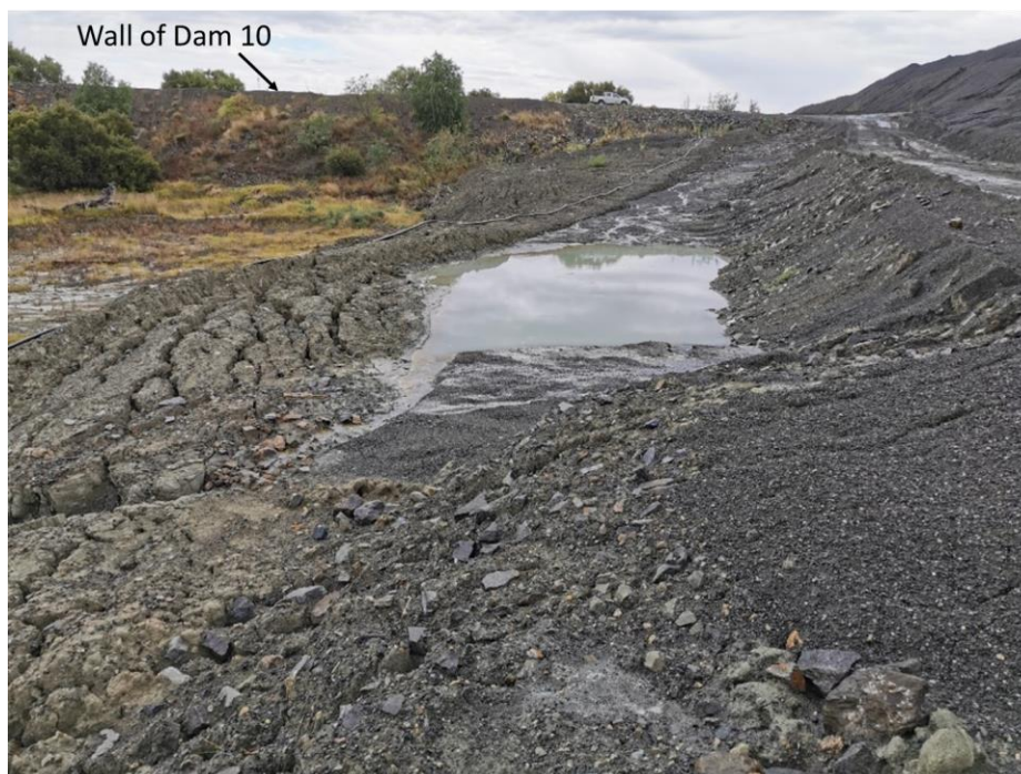
FIGURE 5 ALTERNATIVE VIEW OF LOCATION SHOWN IN FIGURE 4, WITH CRACKS VISIBLE TO THE LEFT AND ACCUMULATED WATER VISIBLE NEAR THE CENTRE. (DATED 21 APRIL 2020.)
