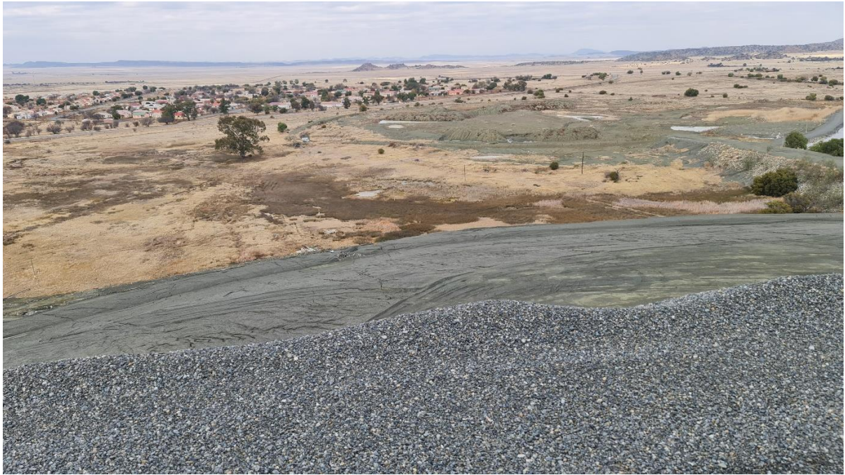
FIGURE 8 SIMILAR VIEW TO FIGURE 6 WITH THE DAM 10 EMBANKMENT VISIBLE ON THE RIGHT, INDICATING CRACKS VISIBLE IN THE BUTTRESS ALONG THE SOUTH-EASTERN CORNER OF THE TAILINGS DAM WALL. (DATED 27 JULY 2022.)
