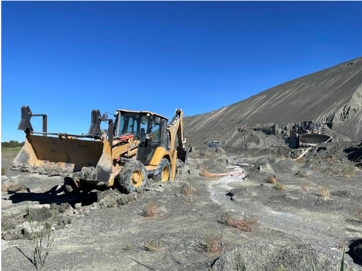
FIGURE 1 WATER LOGGED CONDITIONS ALONG THE SOUTHERN TOE PREVENTED ACCESS BEYOND THE ACCESS ROAD.
