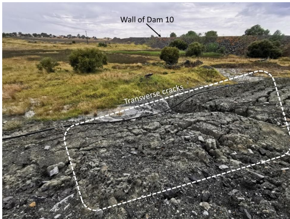
FIGURE 4 TRANSVERSE CRACKS ON SOUTHERN WALL INDICATIVE OF MOVEMENT PERPENDICULAR TO CRACK DIRECTION. (DATED 21 APRIL 2020.)
