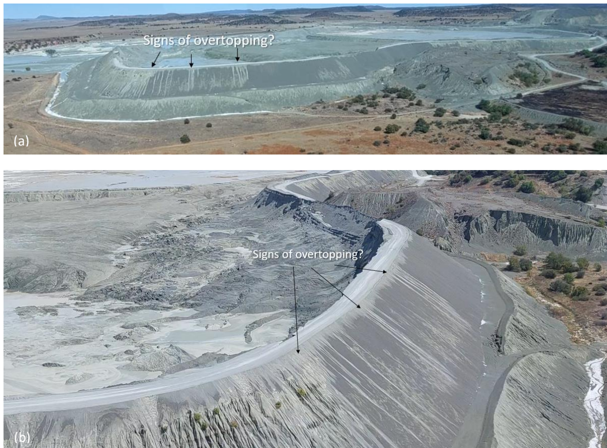
FIGURE 37 IMAGES FROM CELL PHONE FOOTAGE TAKING DURING HELICOPTER INSPECTION ON 12 SEPTEMBER 2022 SHOWING POSSIBLE SIGNS OF LIMITED OVERTOPPING NEAR NORTH-EASTERN CORNER OF DAM (SOURCE: MR A HAVENGA AND/OR MR WM RAMOKOPA).
