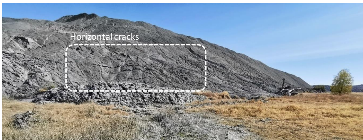
FIGURE 3 WET CONDITIONS ALONG THE SOUTH-EASTERN TOE OF THE DAM WALL. NOTE HORIZONTAL CRACKS VISIBLE ALONG EMBANKMENT SLOPE, POSSIBLY INDICATIVE OF MOVEMENT. (DATED 28 AUGUST 2019.)
